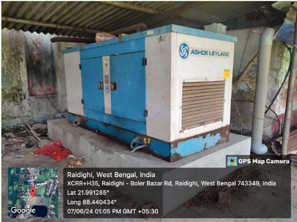
COLLEGE GREEN GENERATOR
