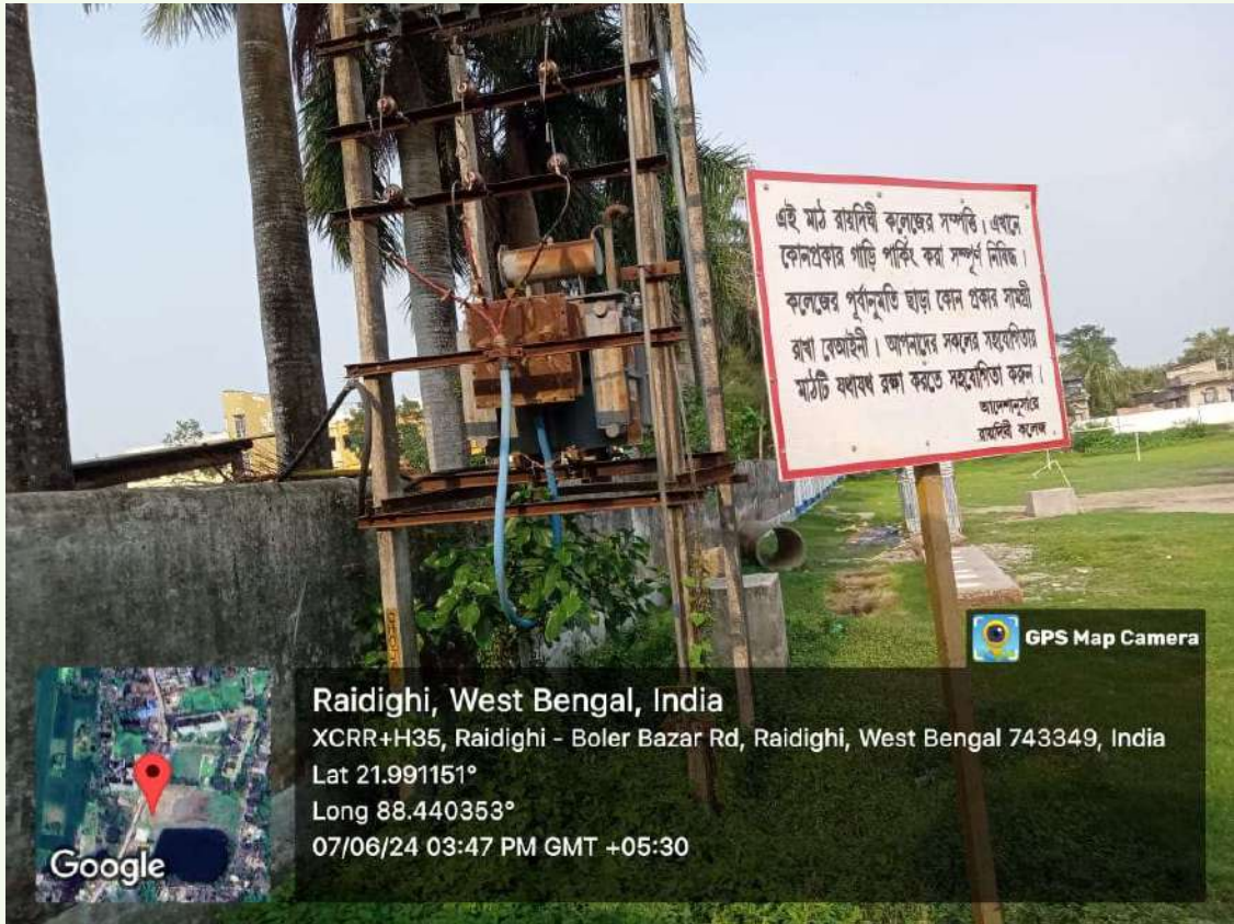
Transformer for dedicated uninterrupted power supply
